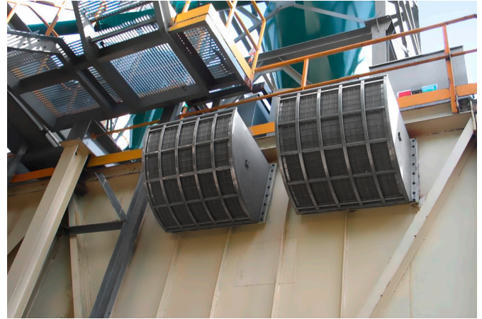
Explosion venting of a chip bunker using the Q-Box to protect the surrounding infrastructure.
